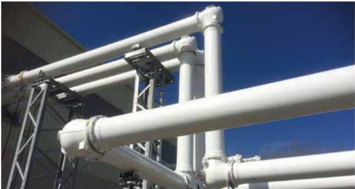
Figure 7. GE – 420kV G 3 GIL solution at National Grid substation in Sellindge, UK
