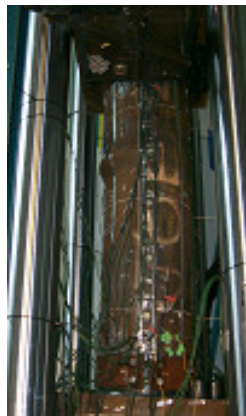
Figure 11. Localized pipe-wall deformation identified by a photo taken from the neutral line 9 o'clock
