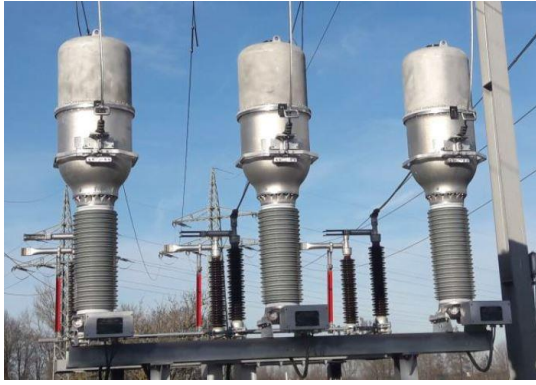
Figure 11: First pilot installation of 123 kV clean air combi transformers in substation Nördlingen (Germany)
