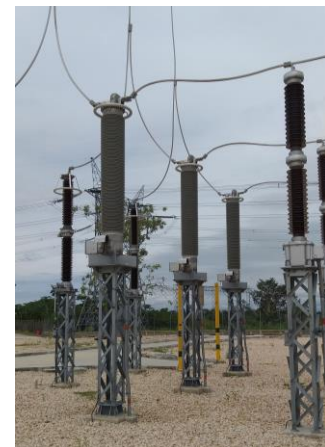
Figure 10: 245 kV OCT installation
