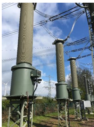
Figure 13: 420 kV clean air voltage transformer installed in TenneT TSO grid.
