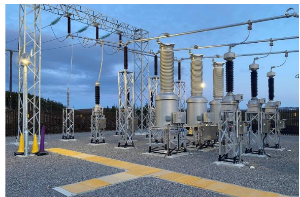
Figure 14: 145 kV, 50kVA clean air Power VTs at Glen Kyllachy substation at SSEN Transmission for connecting a windfarm.
