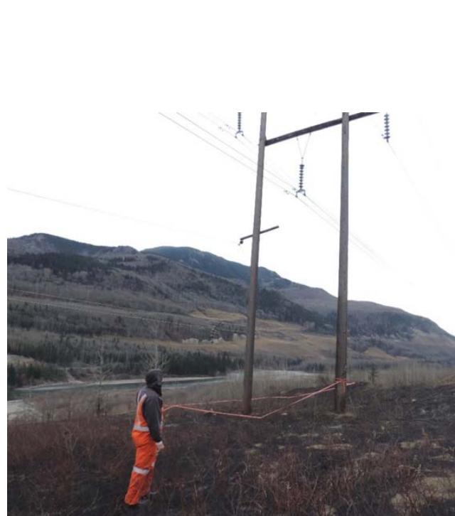
Figure 2: Crossarm Failure Causing Grass Fire
