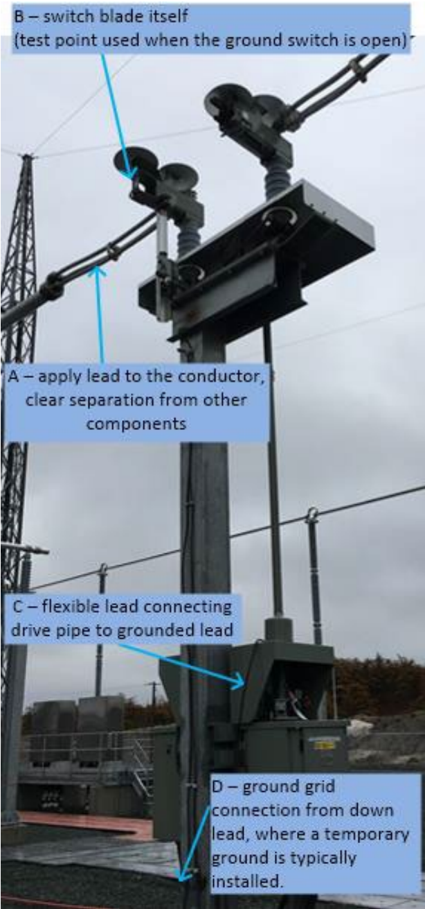
Figure #4 – centre break switch open with a ground switch closed with an explanation of the test
