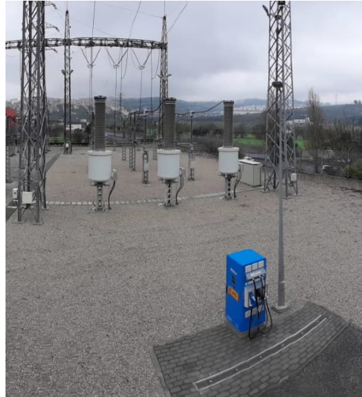
Figure 3: Demonstration Project connected to a 220 kV overhead line in Lisbon area
