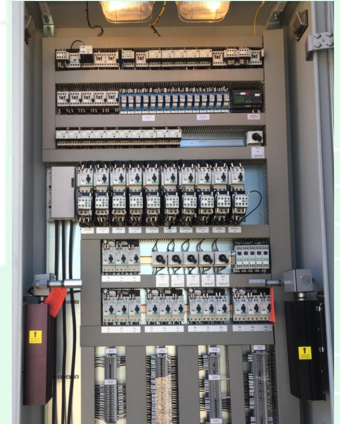
Spare Converter Transformer Cooling Controller: The simplest “in-service” device to test
